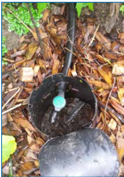
One of the drain outlet valves is covered and soaks into a mulch basin.
