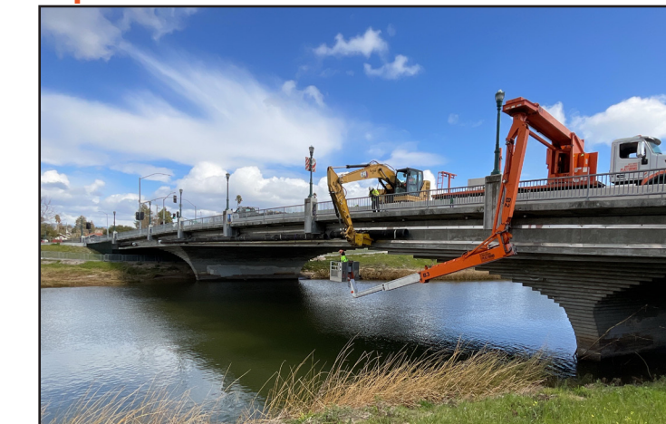
Pipeline advancing over the Laurel Street Bridge in Santa Cruz that will bring the water to the Purification Center.
