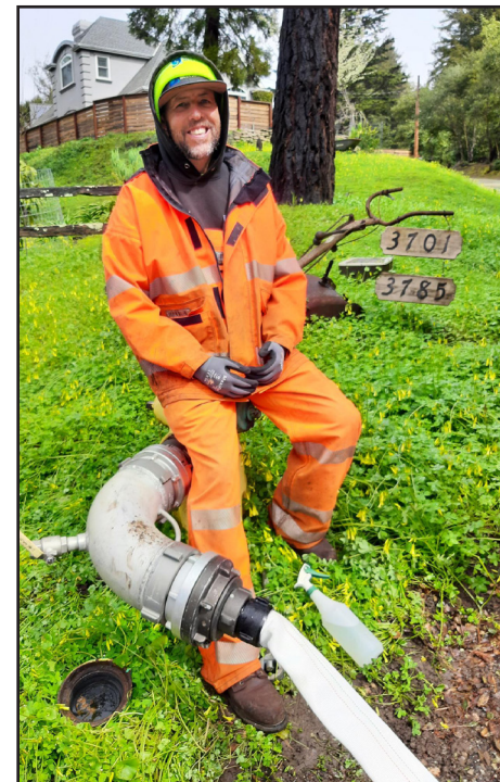
Mark, from our O&M department, with the hose connection to one of the hydrants, that is temporarily providing water to residents.
