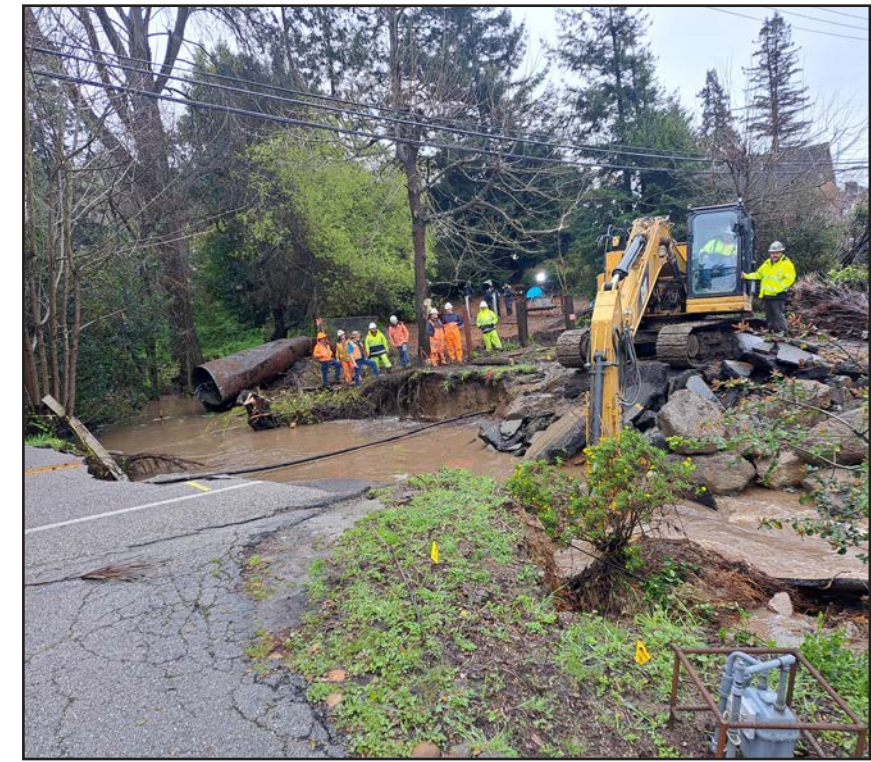
The Bates Creek Culvert in Soquel, off of Main Street, washed out during the March 10, 2023 storm and took our 8-inch main with it.
