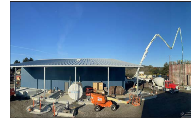
The recycled water purification building at Chanticleer will house the microfiltration and reverse osmosis membranes.
