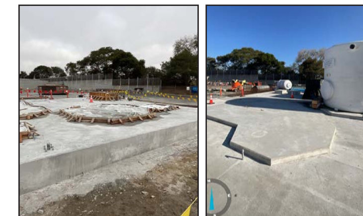
The recycled water treatment facility being constructed at the Santa Cruz Wastewater Treatment Facility.
