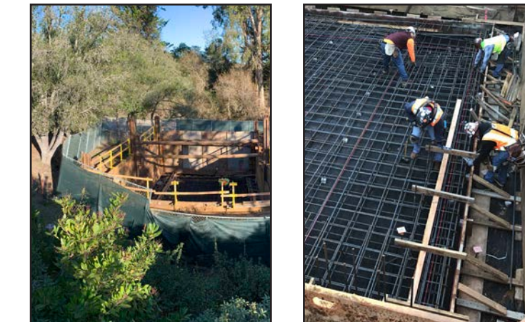
The backwash tank being constructed at the Twin Lakes Church recharge well. Periodic backwashing and rinsing of our well screens will help to maintain performance and optimize replenishing our basin with purified water.
