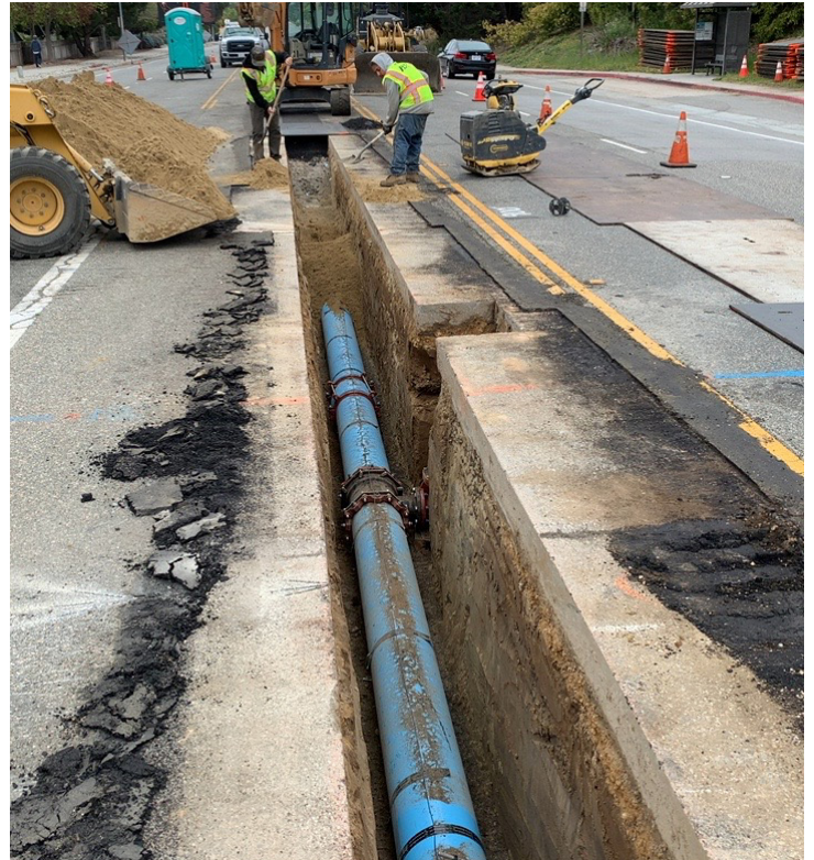
New pipeline is installed along Soquel Drive near Mar Vista Middle School.
