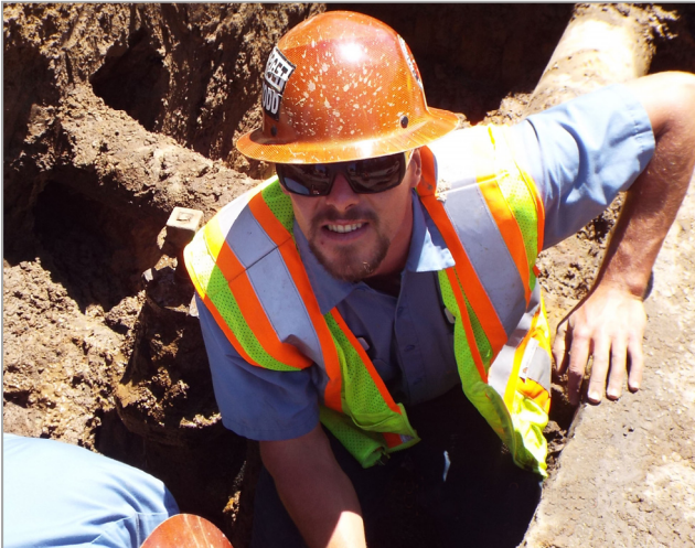
Troy Mumm, one of our District's Construction and Maintenance Workers, fixing a broken water main. Part of the process includes flushing the water main to ensure the pipe is clean and ready to distribute water to our customers.
