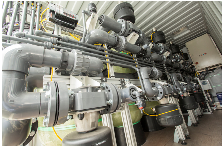
The full-scale treatment system has been constructed by IonexSG at the San Andreas Well, and startup is scheduled for early October.
