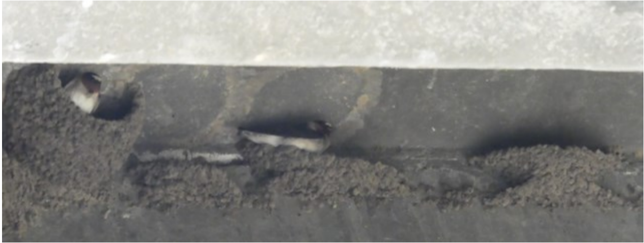
Nesting activity under the Laurel Street Bridge in the areas identified in the first photo.
