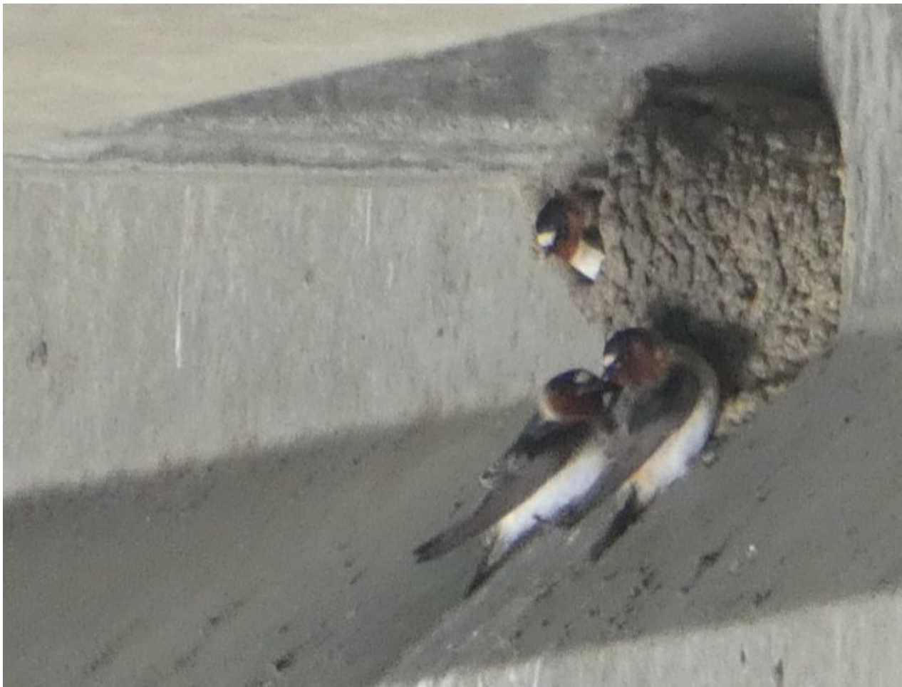
More nesting activity under the Laurel Street Bridge in the areas identified in the first photo.
