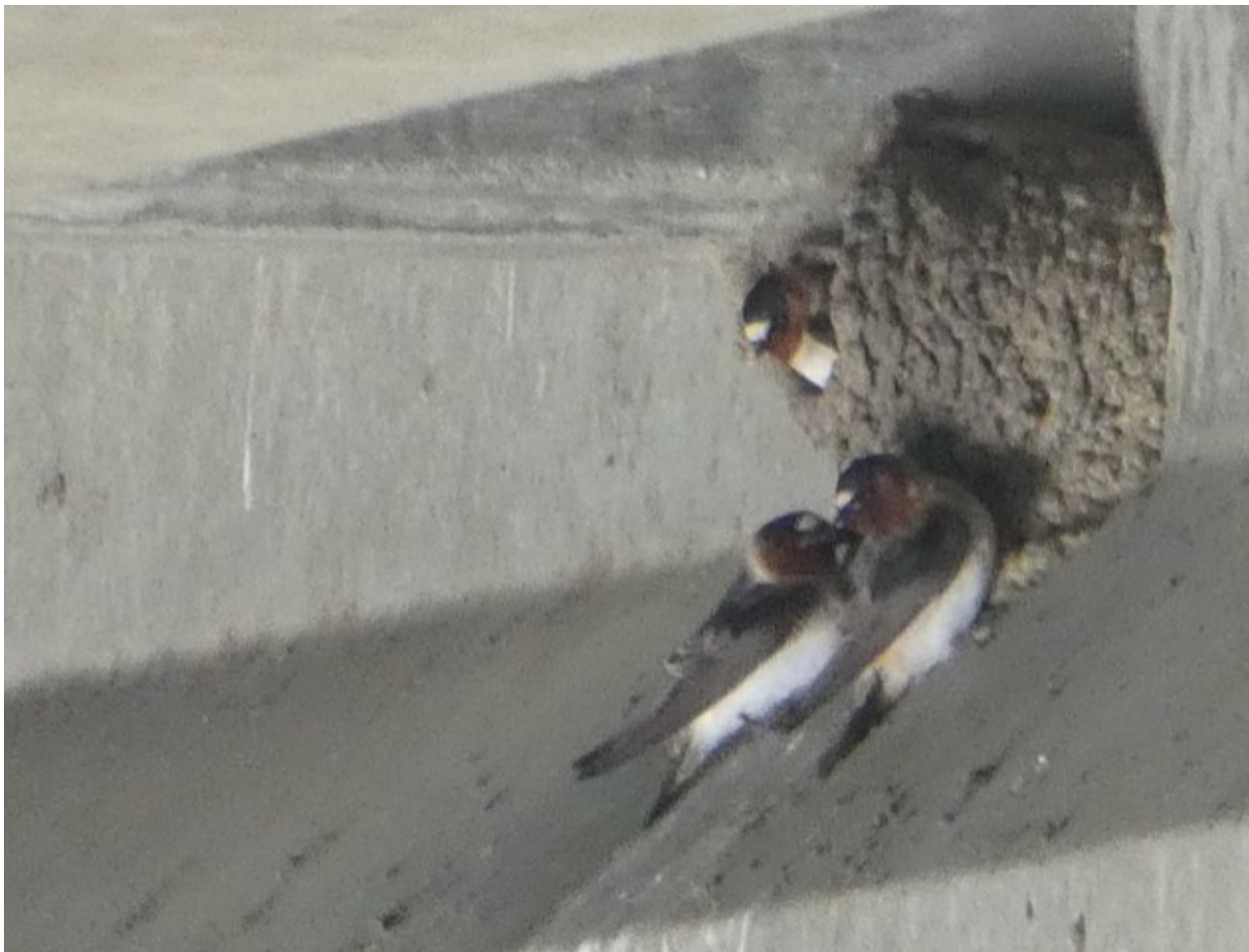
More nesting activity under the Laurel Street Bridge in the areas identified in the first photo.
