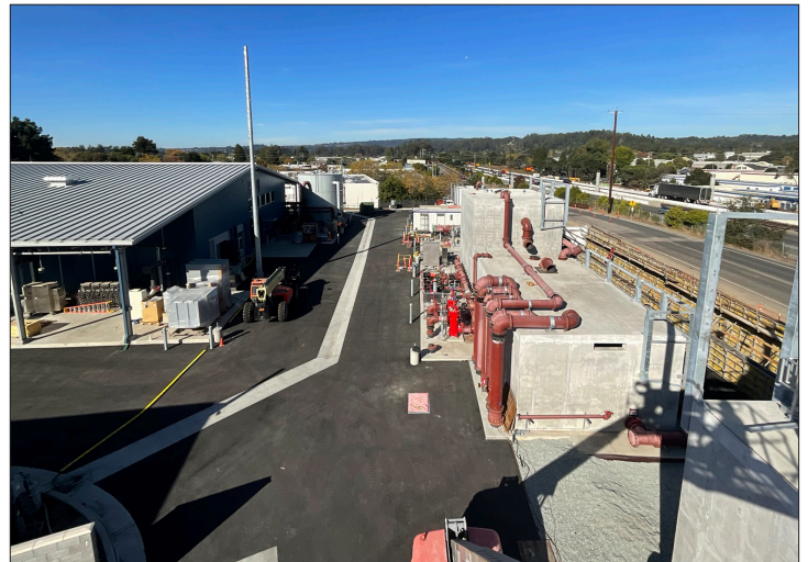
A bird's eye view of the purification building and tanks at the Pure Water Soquel Purification Center.
