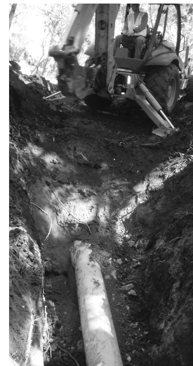
Crews made emergency repairs to restore water service in the Soquel/Maplethorpe area off Fairway Drive.
