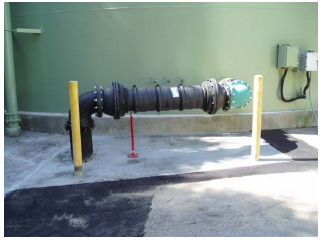
Figure 5 Mar Vista Coupling
