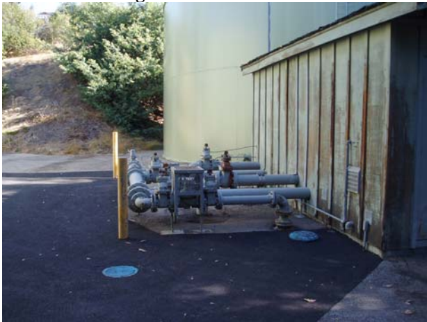
Figure 3 Mar Vista Piping
