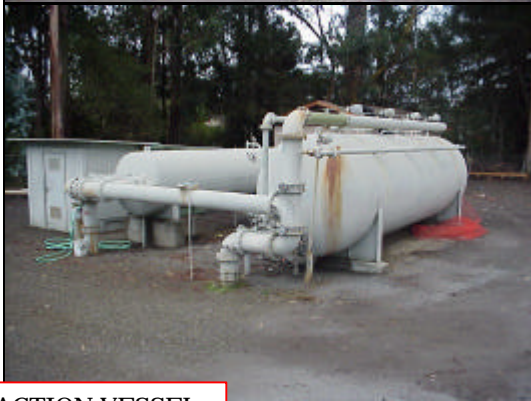
REACTION VESSEL ACCESS HATCH (2)
