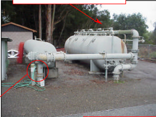
FILTER VESSEL ACCESS HATCH (4)
